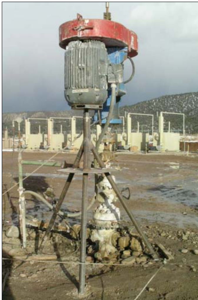
An adequate support corrects the large, vibrating, cantilevered load on this top-drive PCP in the Piceance basin (Fig. 3).
